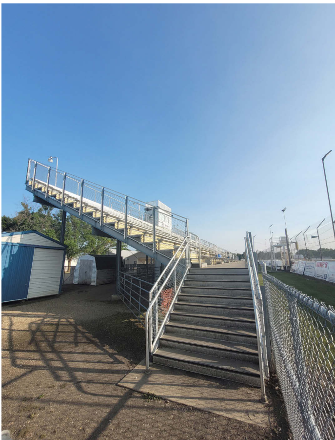
Infrastructure upgrades in Murray County included redoing the grandstands in the fairgrounds in 2008. Wind revenue covered this $452,562 expense.
